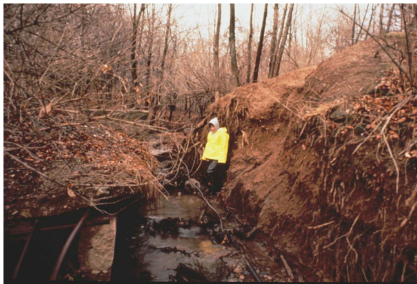
Massive streambank failure after new development (WI DNR photo).
